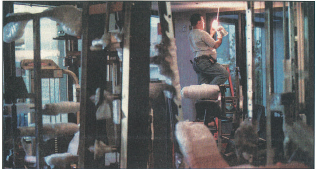
Tony Buffa of PayneCrest Electric Co. installs lights in the workout area at CityPlace 3. Workers also are installing a state-of-the-art system designed by Ascent Corp. to provide wireless Internet access for occupants. (Photo by: Karen Elshout / POST DISPATCH)
