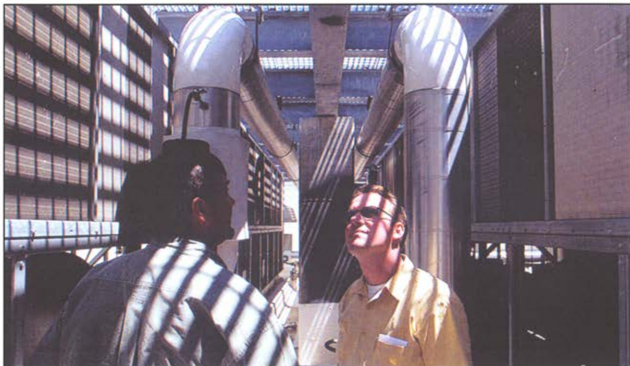
Phil Horstmann (right), president and founder of Ascent Corp., and Mark Moffett, critical systems engineer, look over the air-conditioning units for Savvis Communications Corp.'s data center in Hazelwood. The temperature in the building stays at 68 degrees to keep the computers running smoothly. Horstmann has built Ascent into a multimillion-dollar firm that specializes in advanced technology consulting.
